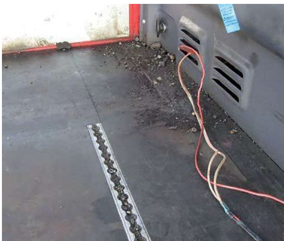
Improper cable wiring by the customer
