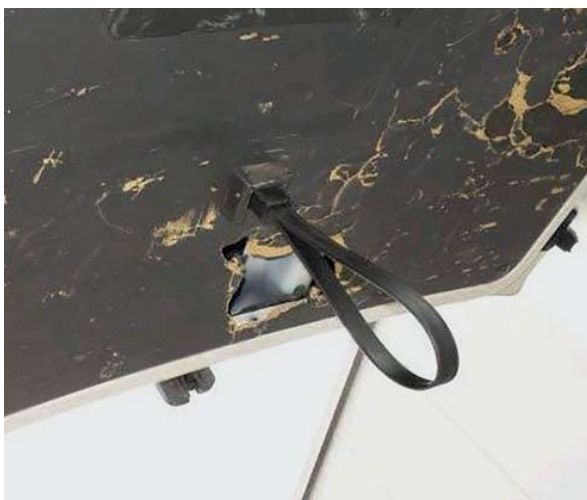
Heavily damaged interior lining
