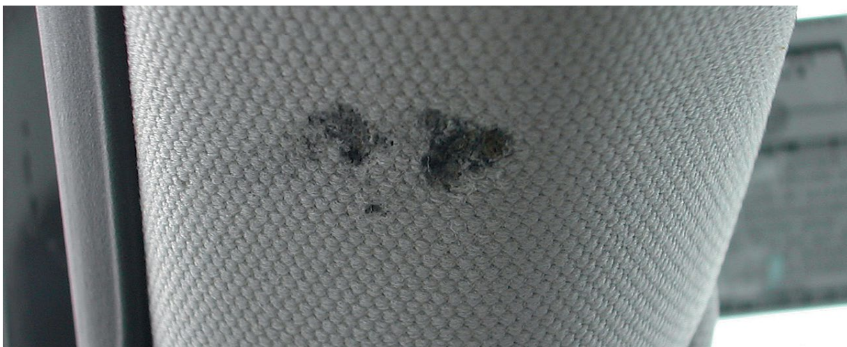
Hole in interior lining
